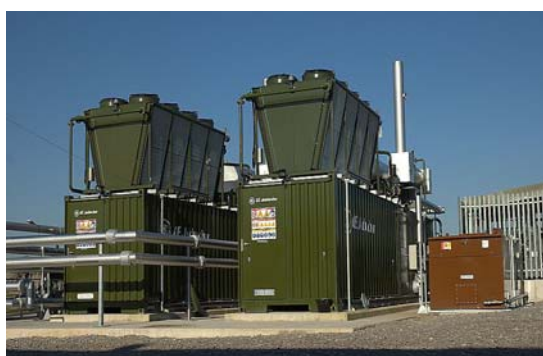
Figure 6 Combined Heat and Power (1MW capacity)
