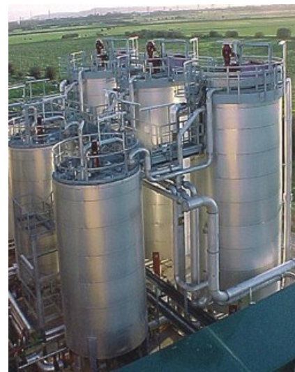
Figure 2 Alpha Biotherm Plant at Ellesmere Port Wastewater treatment works
